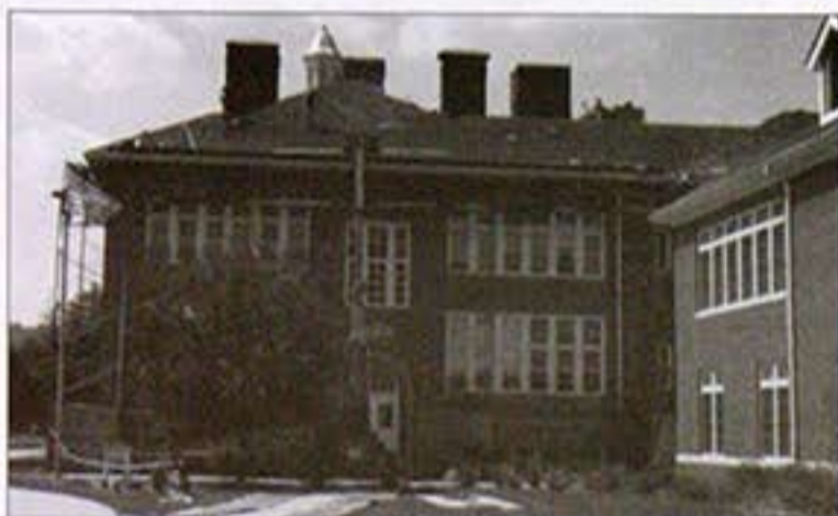
Crews work on the roof of Mount Kisco Elementary School during the waning days of summer to get the building ready for last week's opening.
